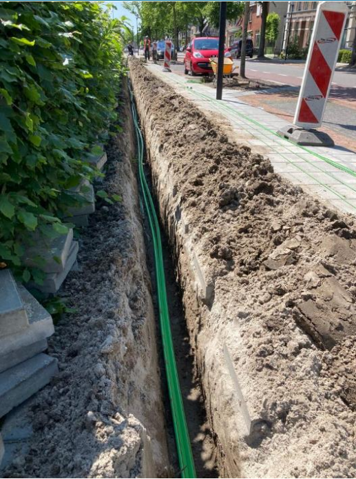
Cityring ducts to POP's + home connections
